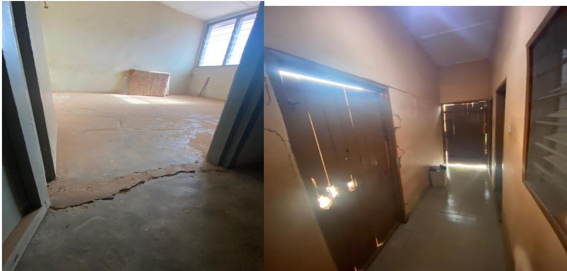
Photos showing a crack floor and corridor of the building
